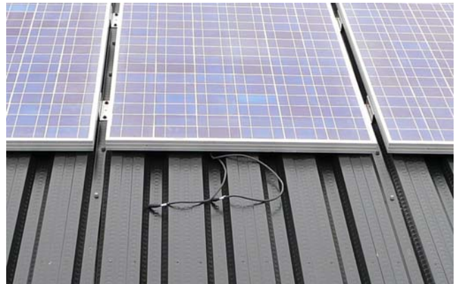
Fig. 2 PV panels on SolarWall® test panel
