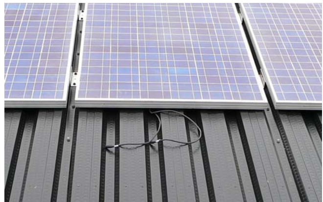
Fig. 2 PV panels on SolarWall® test panel
