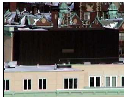
Full south view of the SolarWall® system
