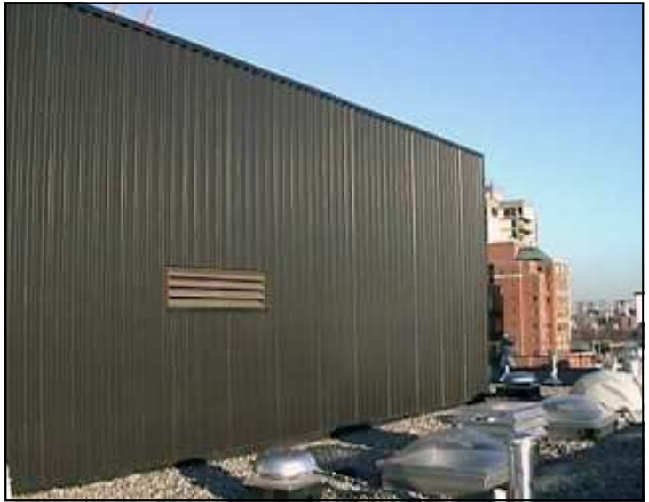
Close up of the SolarWall® system installed on the penthouse mechanical room
