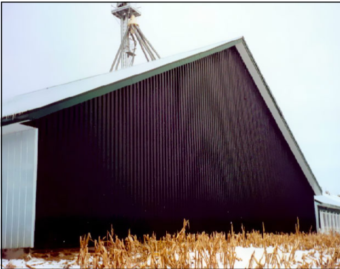
Typical end wall installation with solar heated air distributed above central corridor
